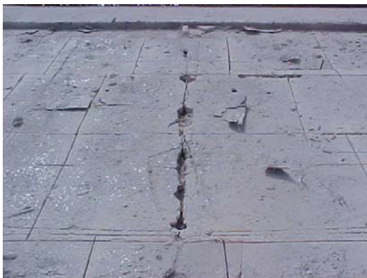
4. Deteriorated Gypsum Deck
